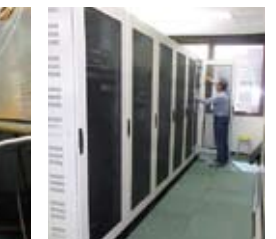
Data Acquisition System
