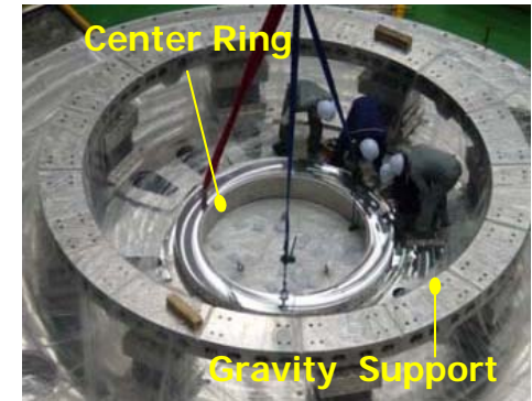
Interface Check between Base and SC Bus-line Duct
