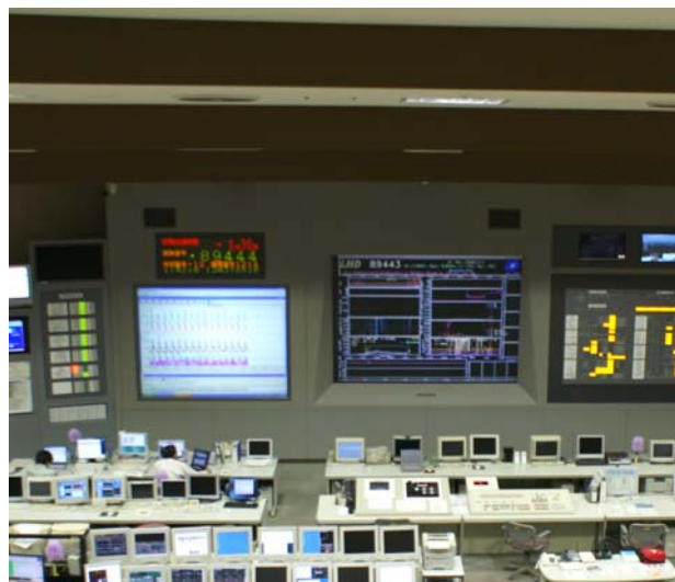
Fig.1 Control room in NIFS
