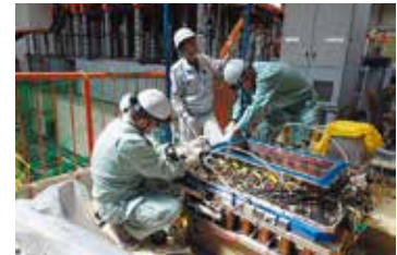
Maintenance of NBI system
