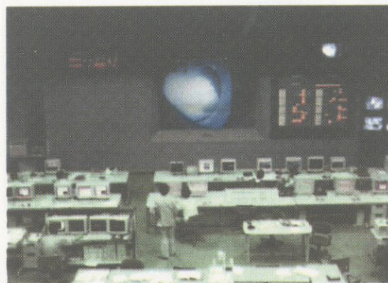
Figure 2: Photograph of LHD Central Control Room
