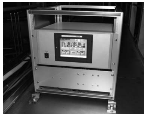
Fig. 2 PLC based control board for the 1.5L-ECH antenna.
