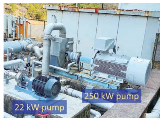
Fig. 7 Cooling water pumps
