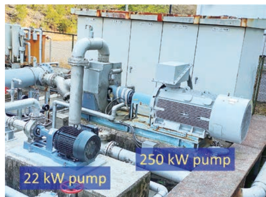
Fig. 7 Cooling water pumps
