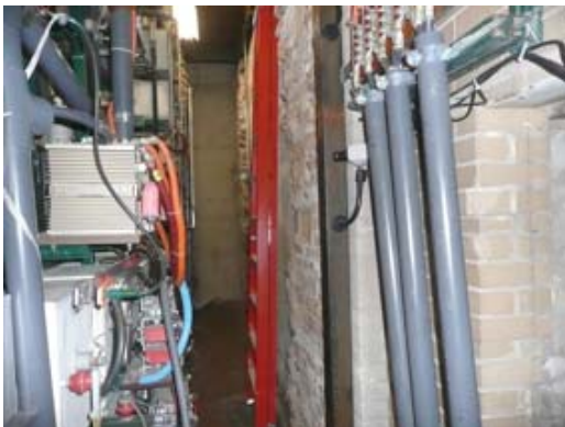
Fig. 26. Narrow passage in the capacitor bank area.
