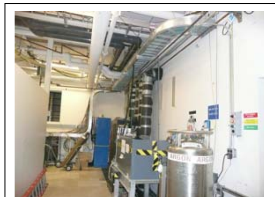
Fig. 8. A stepladder and a gas cylinder on a carrier are kept on a passage.
