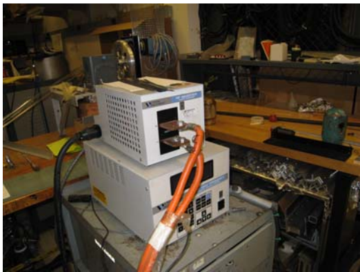
Fig. 10. Current terminals without protecting cover.
