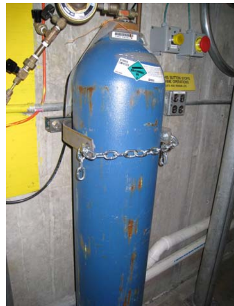
Fig. 23. Gas cylinders with one binding.
