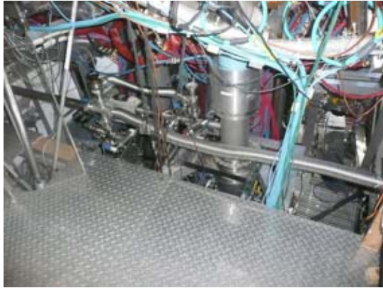
Fig. 31. Periphery of underground pit without toe-boards.
