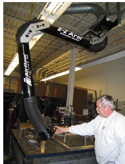
Fig. 12. An air exhauster in the machine-shop.
